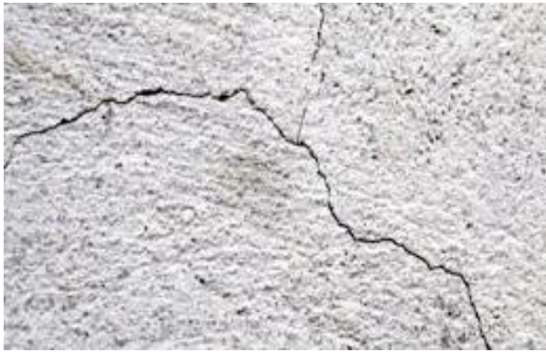
Figure 1. Shrinkage cracks in wall
