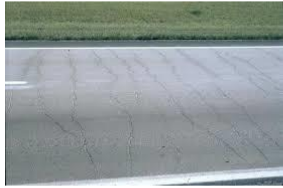
Figure 2. Shrinkage cracks in Pavement
