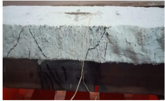
Figure-12: Minor cracks developed in slab(CB1)
