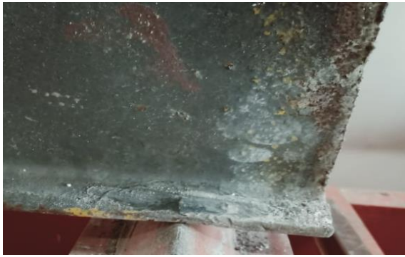
Figure-11: Little buckling of flange at support (CB1)
