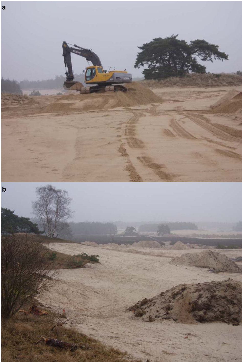
Fig. 10: Management measures carried out. a: topsoil removal at the borderline between dry heath and drift sand in 2009. b: sieving machine in action with piles of sand left after the sieving.
